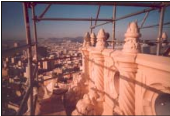
The portholes and spiral columns were cast to match the original design. All brackets were supported with stainless steel tubes and formed chairs. All work was done off of a cantilevered staging.
