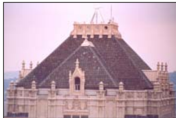
All finished work was sealed and painted to match historical drawings and was completed prior to staging removal.
