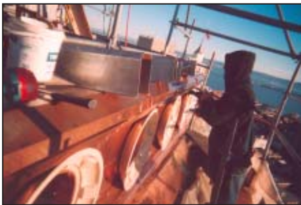
The upper “Crow’s Nest” roof had considerable decay and lost brackets. The entire wall area was reframed and covered with plywood prior to installation of copper work.
